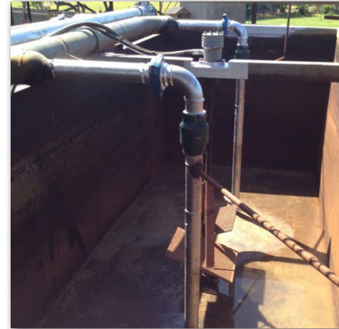
Mixing tank with hydraulic paddles
